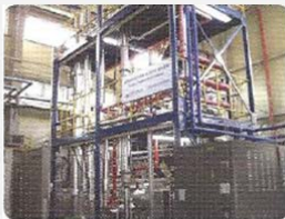
Ammonia CO2 Removal Device
