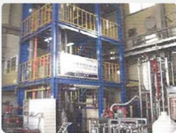
Dry sorbent CO2 Removal Device
