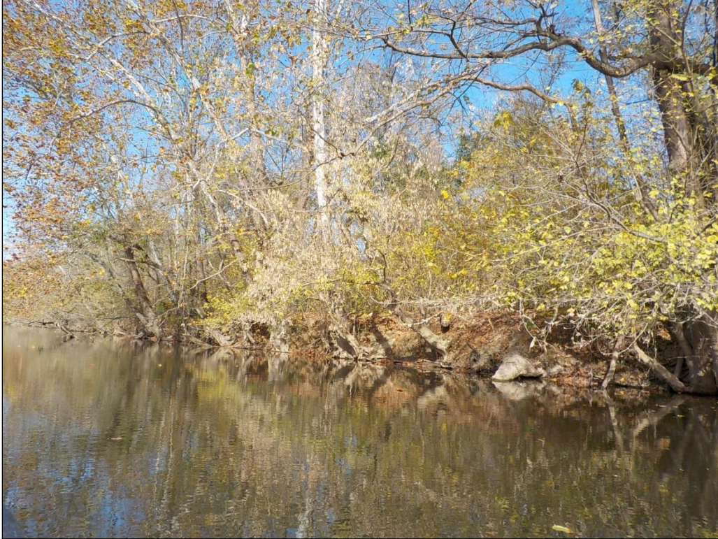
Photograph 1 – Southwestern shoreline of Daniel’s Island (note erosion), view N
