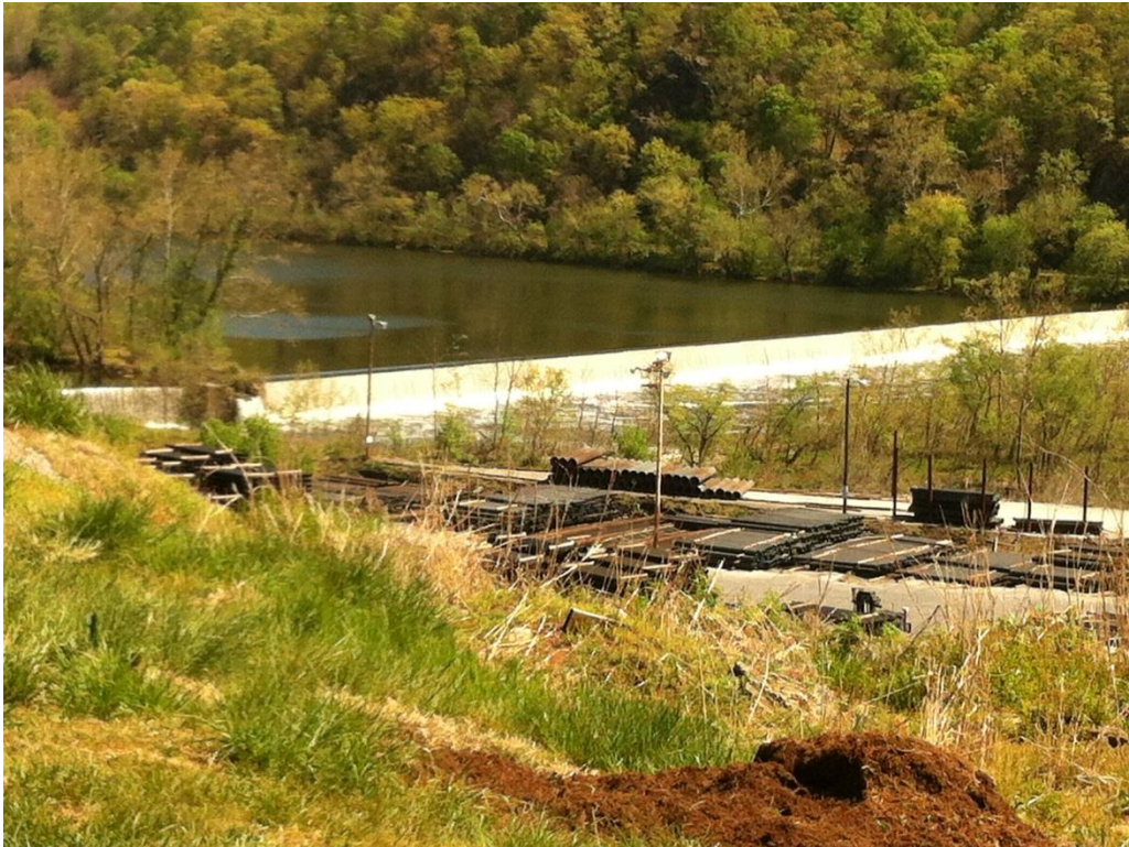
Photo 20 – April 20, 2016 Scott’s Mill dam Viewed from North Side of Norwood Street (Note Pipe Storage Area)
