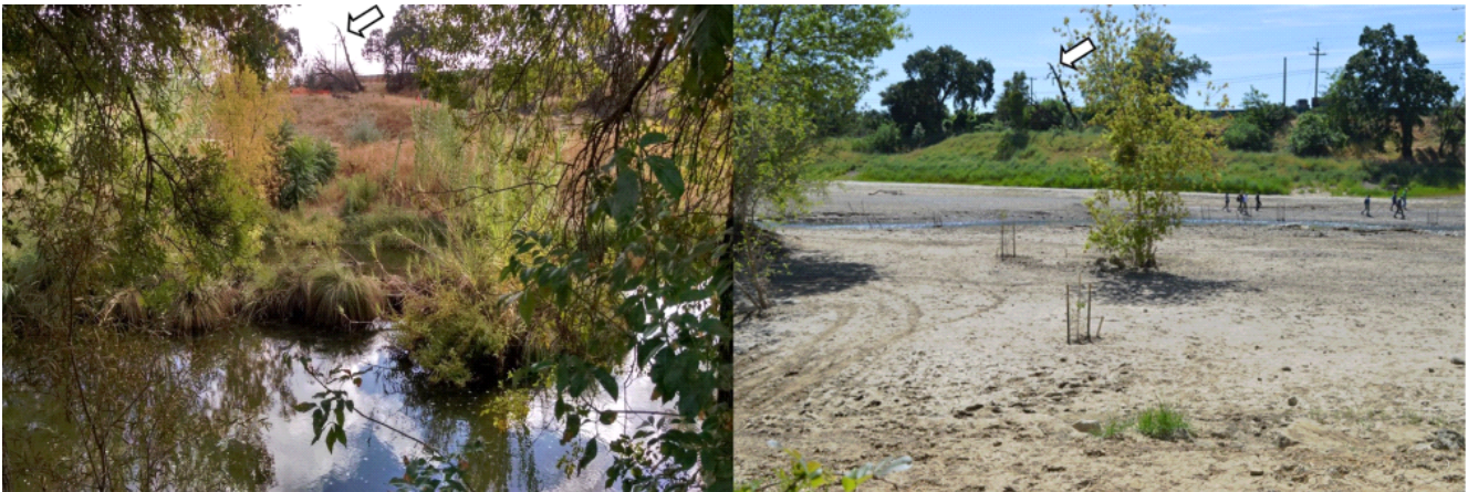
Fig. 1 - Recent “Before and After” photos following bulldozing and leveling of a rich riparian floodplain habitat.
