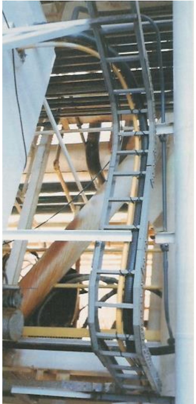
Glass-Steel cabletray and channel tray systems located on offshore platforms in the Pacific Ocean have survived severe storms and salt air and have given trouble-free service.
