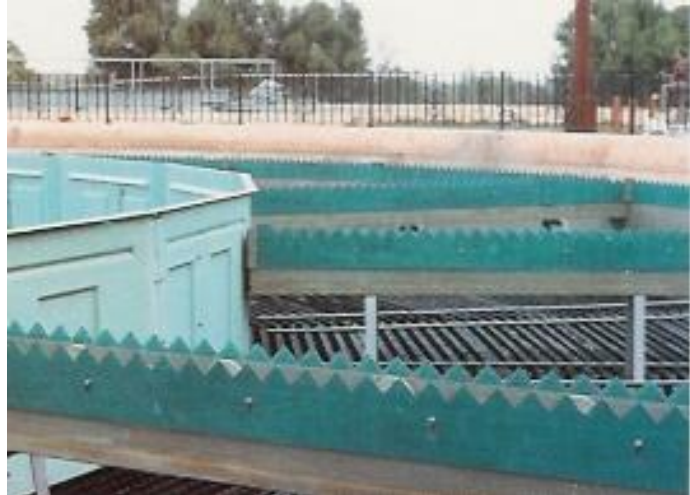
Fiberglass circular troughs with fiberglass weirs, scum baffles, and mounting brackets were installed in three 140' diameter clarifiers at the Laredo, TX Municipal Treatment Plant.
