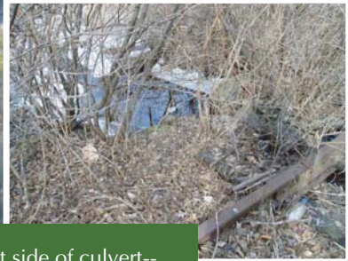
East side of culvert blocked by debris
