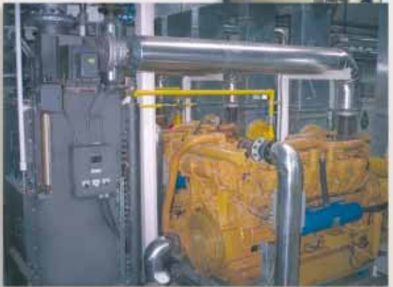
GOLD & SILVER MINE, Eskay Creek, British Columbia. (3) Model HRSR-316A26CSP Recovering Btu from (3) Caterpillar 3512, 900kW diesel engines. Reducing each 870°F @ 2,100 SCFM to 417°F. Raising 265 GPM 50% ethylene glycol from 187°F to 197°F.
