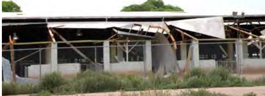
Wind damage, County Fairgrounds, 2012
