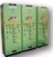
Wired and Bare Panel
