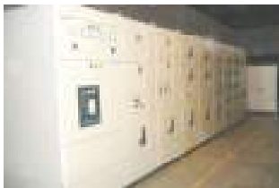
Drawout type MCC/PCC
