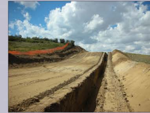
Dated features are frequently discovered in settings like this, a bladed right-of-way. Clearly, there is a lot more disturbance in the bladed surface than in the trench itself, which likely biases discovery toward the upper 30 – 50 cm, or toward recent/shallow finds. However, we could not find clear evidence for this bias in our analysis.
