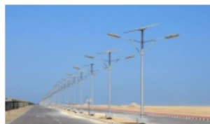
Solar PV LED Street Lighting
