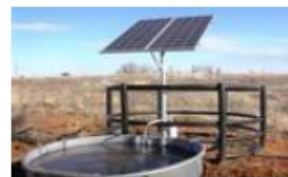
Solar PV Water Pumps
