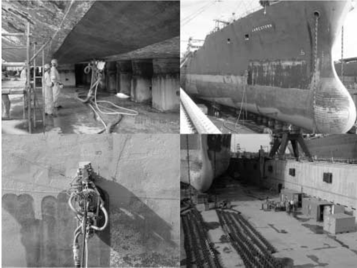
Fig. 11. Clockwise from top left: under-hull operation; sweeping the bow; dockyard with pump and vacuum containers; stripping failed coating.
