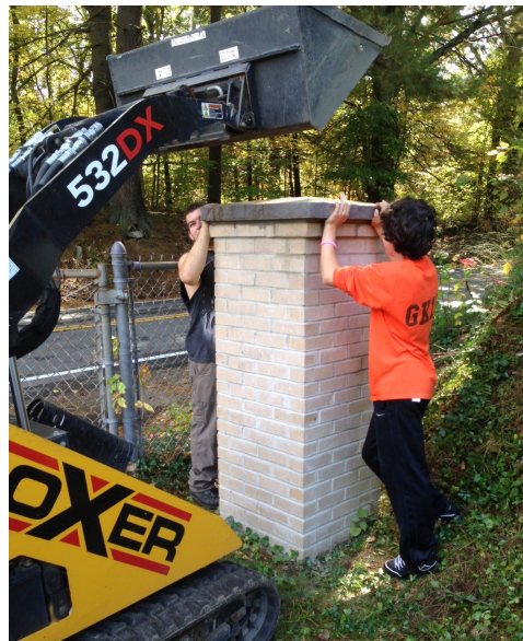
Jimmy Kosidlo, left, and Ian Ford-Hunt provide visual guidance to ensure proper placement of the capstone on top of the left pillar of the new rear dirt road entrance to the cemetery.
