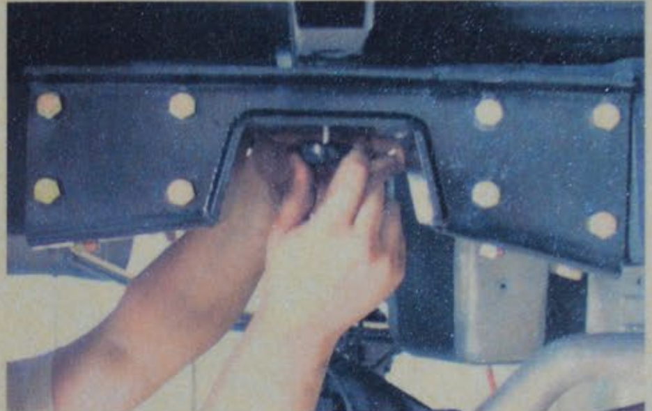
11. Using the supplied hardware, the C-notch plate was bolted on using Grade 8 bolts, and checked for alignment and angle.
