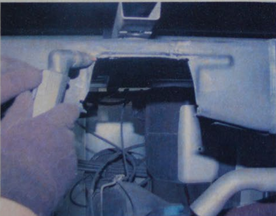
10. Moving to the rear, Mike supported the axle with a jack, removed the U-bolts, and marked out the area of the frame to cut using a plasma handheld cutting torch for the C-notch. He used a plasma cutter to cut the frame.
