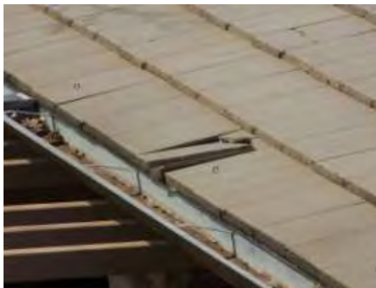
Broken Tile - Typical
