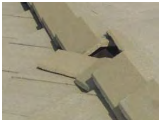
Broken Tile - Typical
