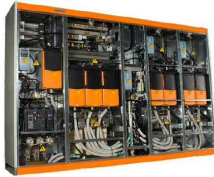
Figure 5: Four Quadrant Converter, courtesy The Switch
