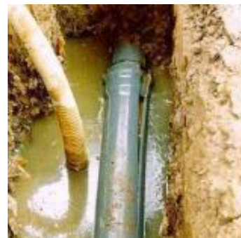
Figure 9: PVC Cracking (WSAA [6])
