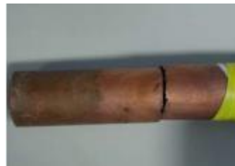
Figure 8: Copper Cracking Without Corrosion (WSAA [6])
