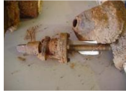
Figure 15: Corroded and Cracked Underground Valve (WSAA [6])
