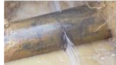
Figure 6: Cast Iron Cracking Without Corrosion (Figs. 6 – 15 reprinted by permission of WSAA [6])
