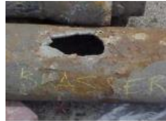
Figure 7: Ductile Iron Cracking and Corrosion (WSAA [6])
