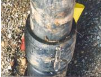
Figure 11: HDPE Electrofusion Joint Leakage (WSAA [6])
