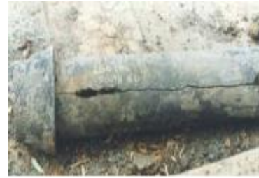
Figure 5: Cast Iron Cracking and Corrosion (Figs. 5 – 15 Reprinted by permission, WSAA [6])
