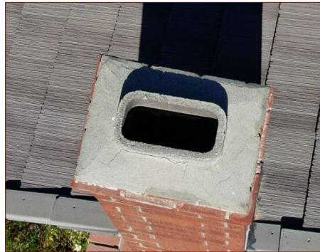
Missing spark arrester
