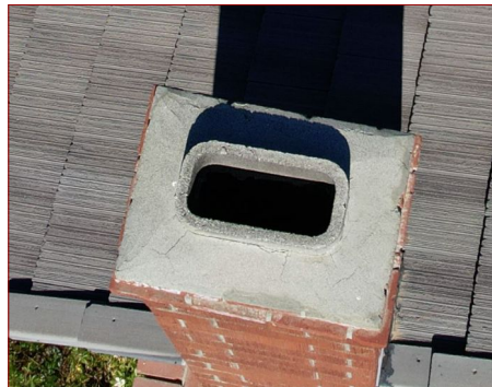
Missing spark arrestor
