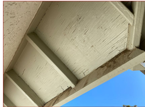
Dry rot observed
