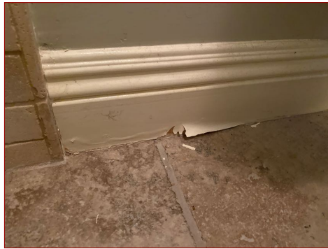
Bathroom 2 - Moisture damage observed
