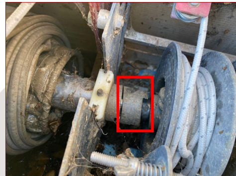
Coupling not engaging to close
