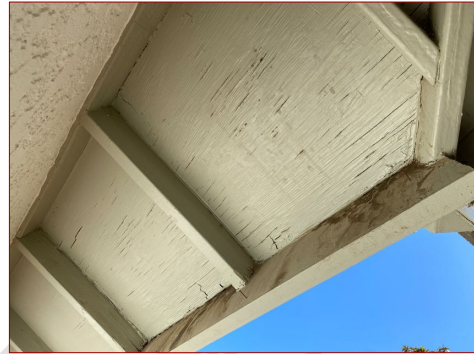
Dry rot observed
