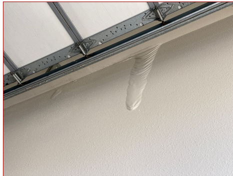
Shop - Evidence of leakage
