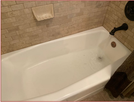
Bathroom 2 - Slow to drain
