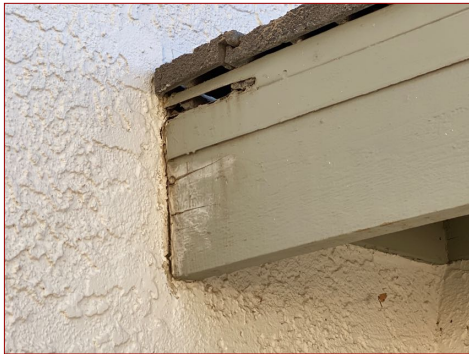
Dry rot observed
