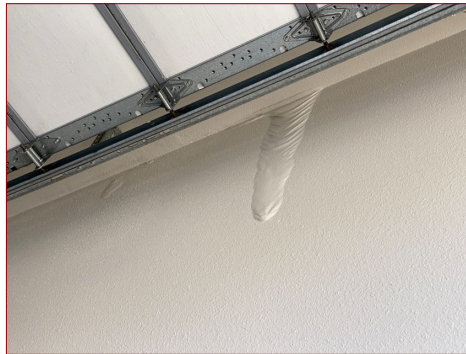
Shop - Evidence of leakage
