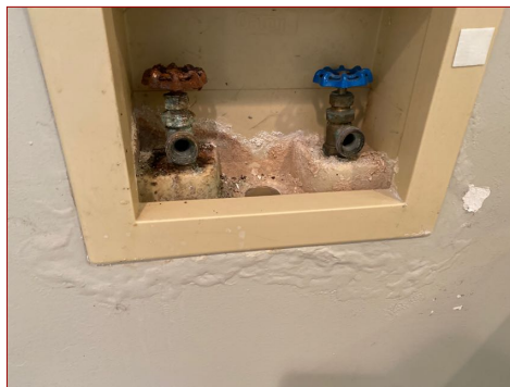
Corrosion/Evidence of leakage
