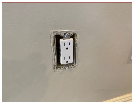
Bedroom 4 - Missing cover
