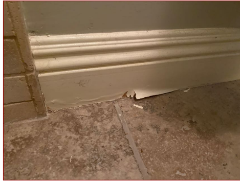
Bathroom 2 - Moisture damage observed
