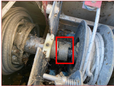
Coupling not engaging to close
