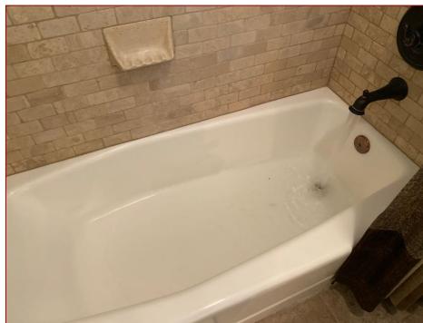
Bathroom 2 - Slow to drain
