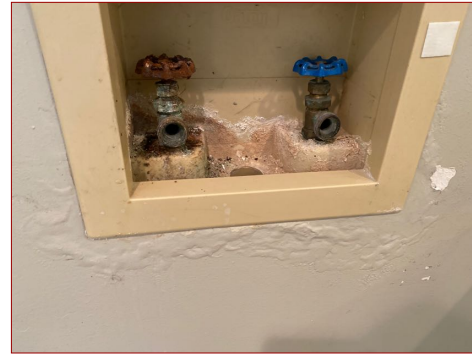
Corrosion/Evidence of leakage
