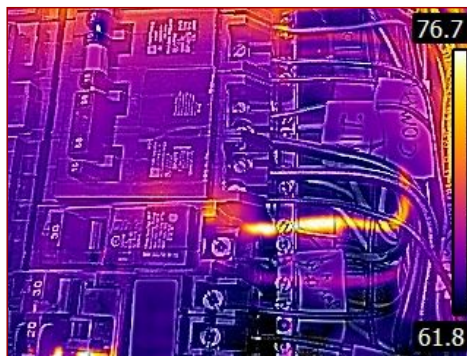
Overheating wire observed
