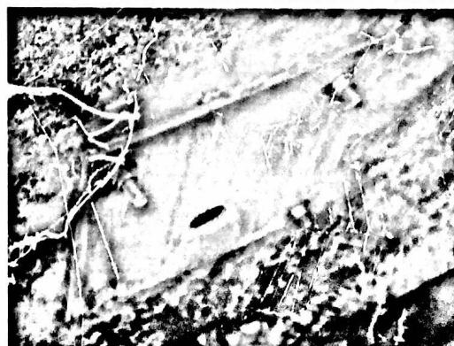
Fig. 8 A typical orifice control plate inside a wet pond control structure
