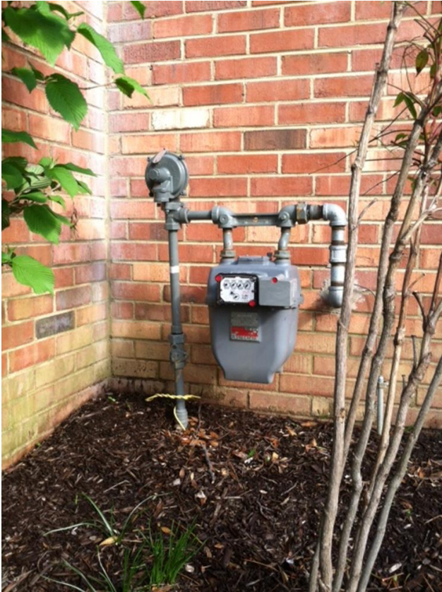
Tied in meter bar with meter
