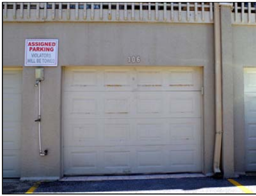
garage garage with automatic garage door opener
