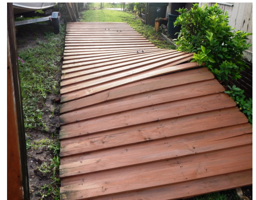
Wood fences took a beating. Note: The City has suspended the requirement for permits for fence repairs for 90 days after the storm
