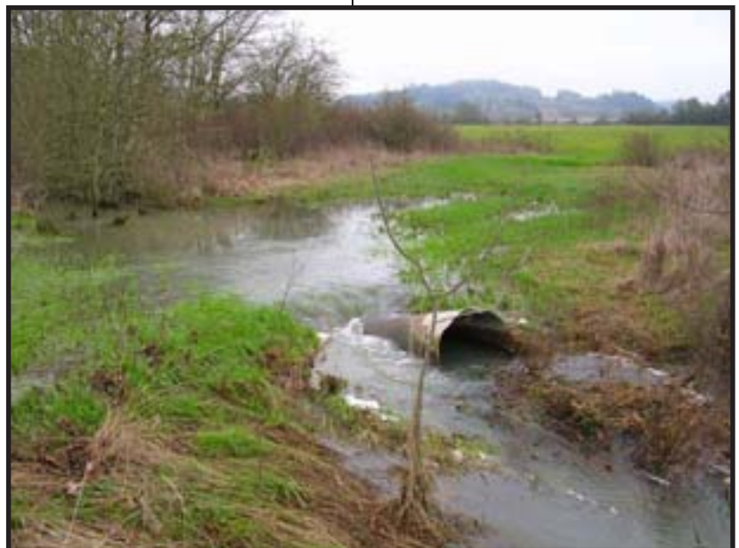
One of the culverts along the East Branch of Coyote Creek to be replaced
