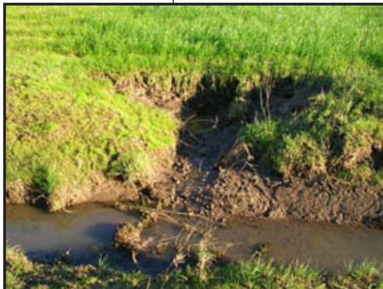
Slumping along Coyote Swale
