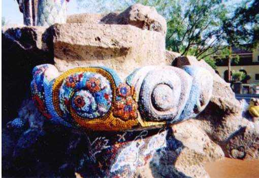
Fountain Efflorescence Removal
