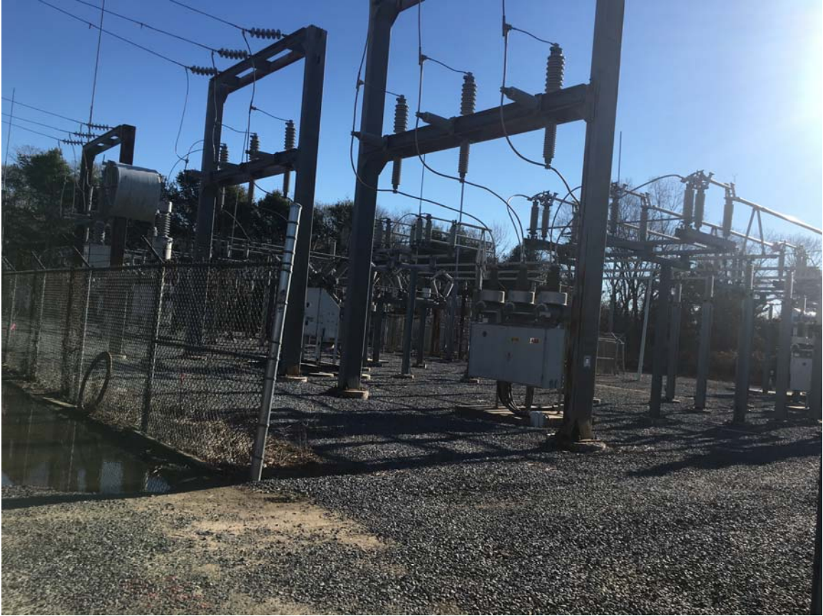
Photograph No. 8: Ground-based transformers, located within the central eastern portions of the subject property.
