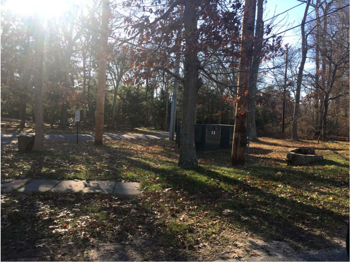
Photograph No. 7: Two pad-mounted transformers located on the eastern portions of the subject property, along Cove Hollow Road.
