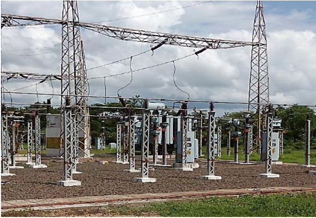
Figure 1. Traction Substation Configuration [7]
