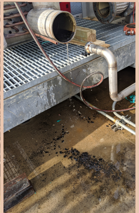
Descaling and Winterization
