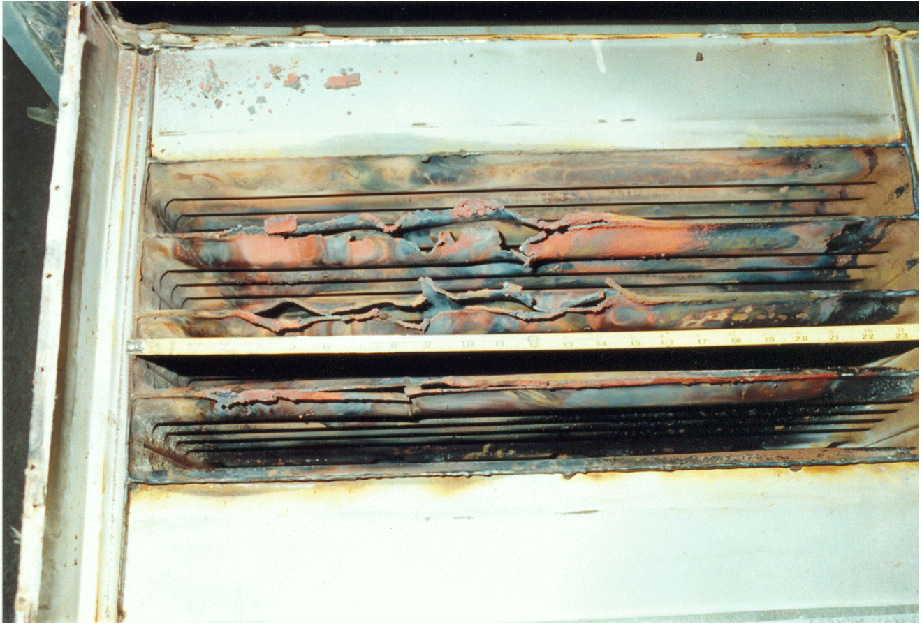
Photo Seven: Major failure of heat exchanger.
