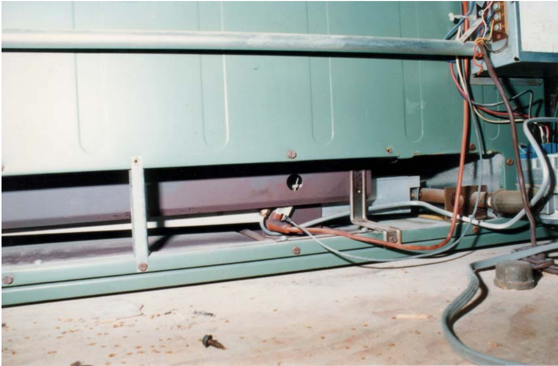
Photo Two: Combustion air intake port at bottom edge of furnace housing.
