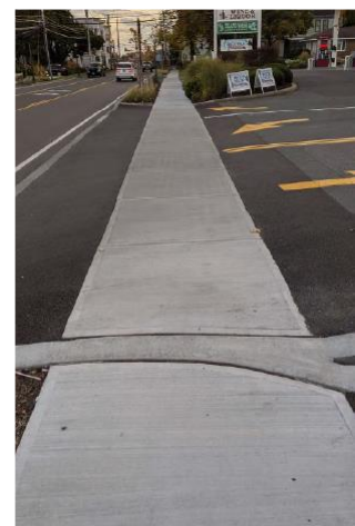
Figure 7. Example of a pedestrian sidewalk that continues through driveway to prioritize pedestrians.
