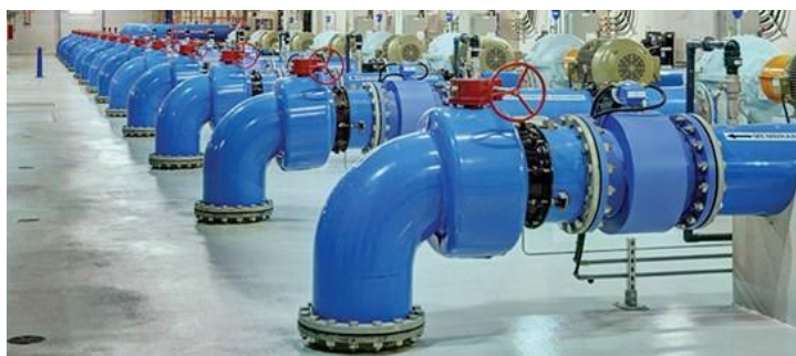
GWD Distribution System Testing
