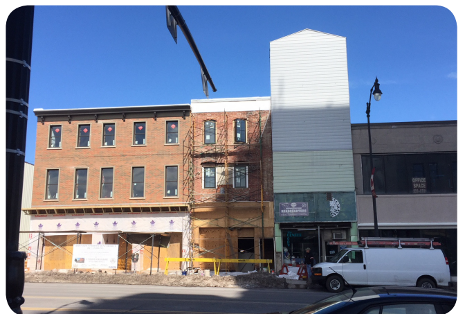
CAN DO began renovations to the 21-23 W. Broad Street property, which is planned to become the Broad & Barrel, a new restaurant and brew pub. We also began facade renovations on the adjacent 19 W. Broad St. property.
