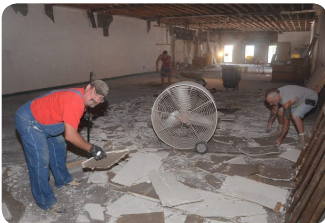
A blighted building (13-15 W. Broad St.) was donated to us and we raised funds to undertake Phase One renovations, which were completed in 2017. This building is planned to become a new business incubator.
