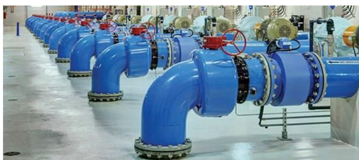
GWD Distribution System Testing
