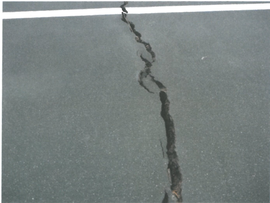
Tennis court cracking
