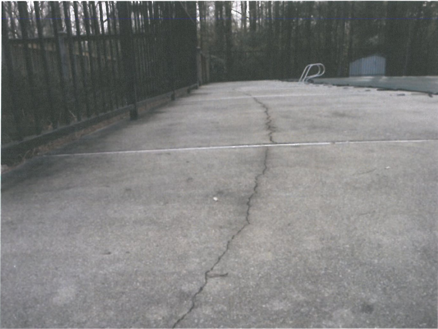
Cracked pool decking surface
