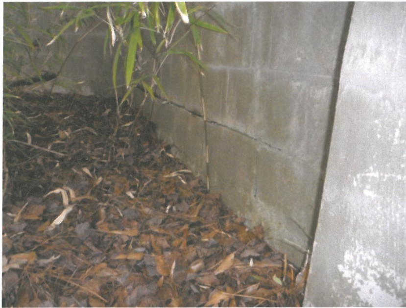
Foundation crack at rear of Entrance Monument
