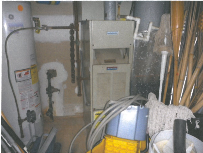
Aging clubhouse furnace
