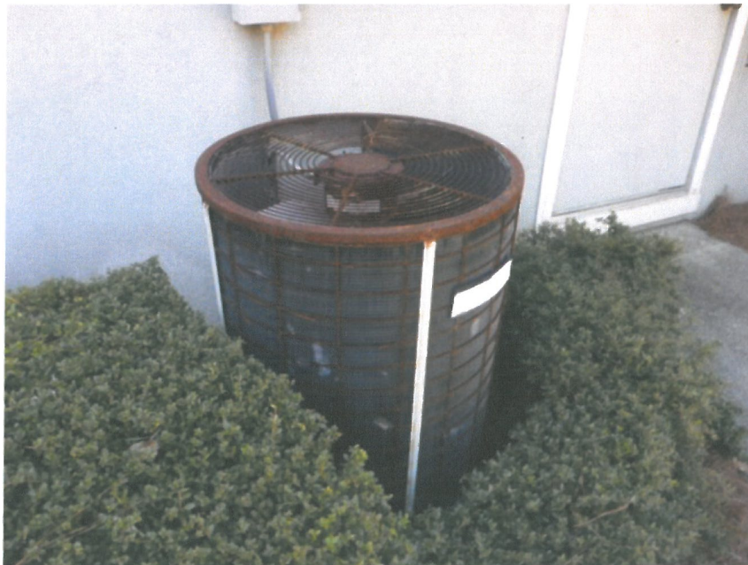
Aging Condensing unit
