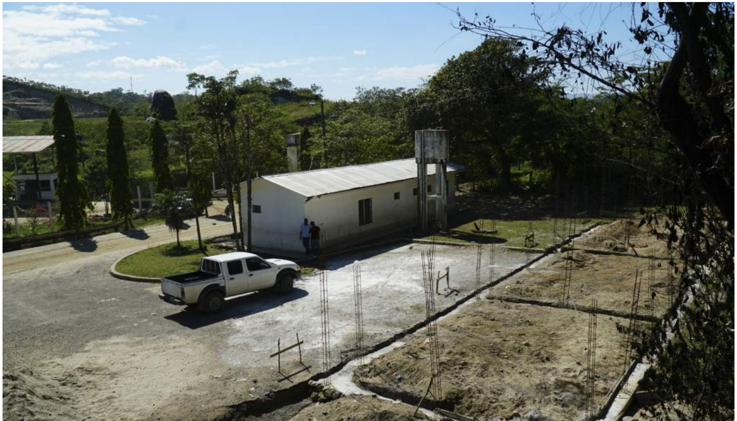
The parents helped in the construction of the foundations of the three classrooms; They will be ready by half a year.
