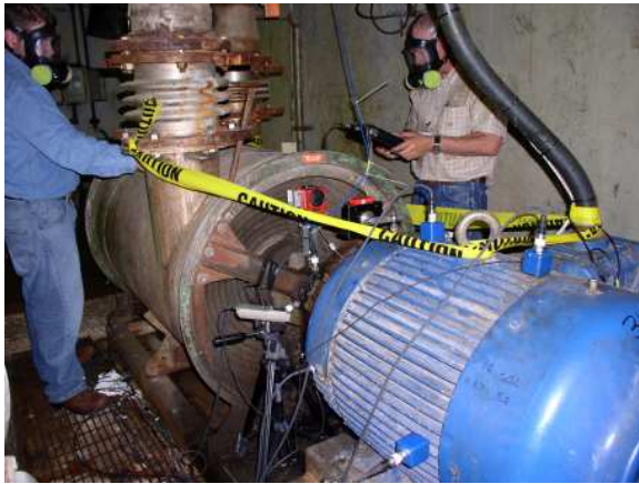
Figure 36. Laser Alignment Equipment, Luduca Permalign Ref 7 , Installed on the Motor and Blower.
