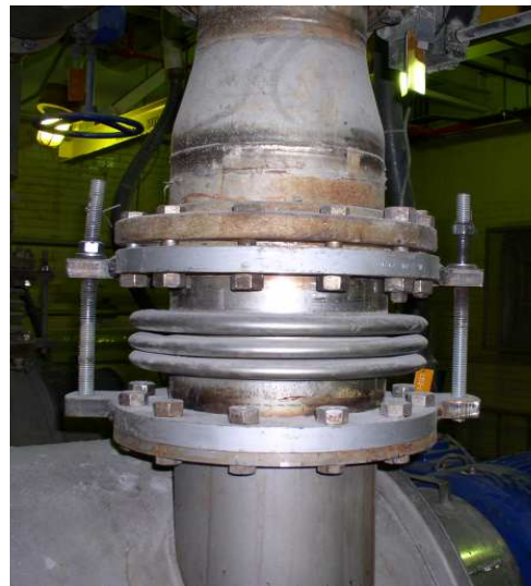
Figure 11. Blower LS 10 Blower Discharge Connection, Bellows Collapsed.
