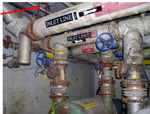
Figure 12. Piping Connected to Blowlers, Blower DB 19 Shown.
