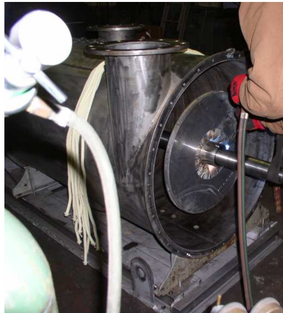
Figure 49. Reassembly. Torch Used to Heat Impeller Hub Prior to Sliding Into Position.
