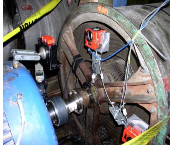
Figure 13. DB 19 With Laser Alignment and Vibration Sensors Attached.
