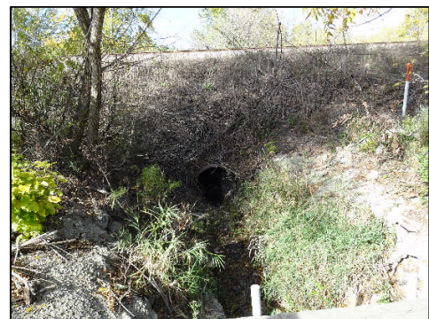
48 inch culvert under of C.-P.R.R tracks, from Gitzlaff side facing west, spring, 2013
