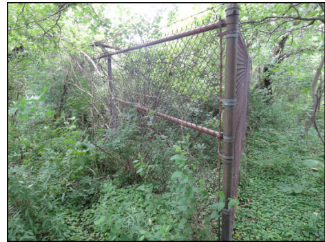
Maintenance yard fence blocks access to north side of Gitzlaff
