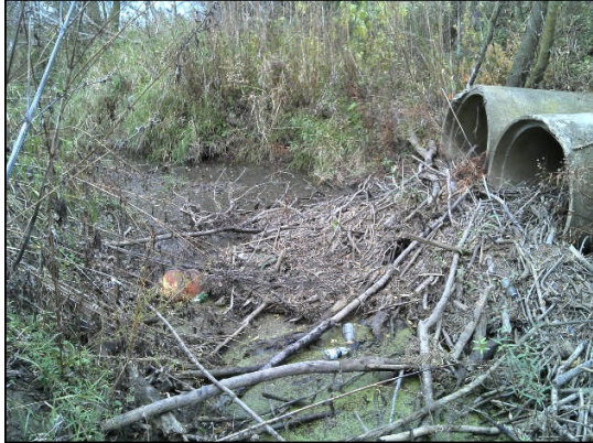
Woody debris under of Union-Pacific RR tracks, on west side of tracks fall, 2013
