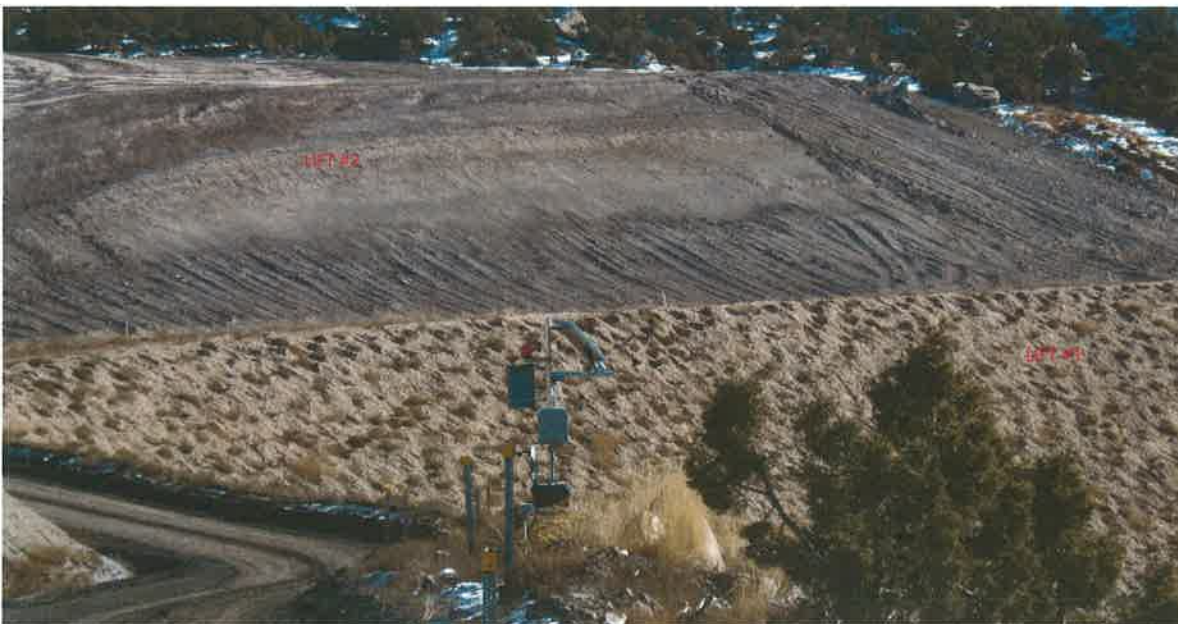
SCA#2 Ash Landfill – lower face looking easterly Lift #1 covered and seeded, vegetation is growing. Lift #2 in process
