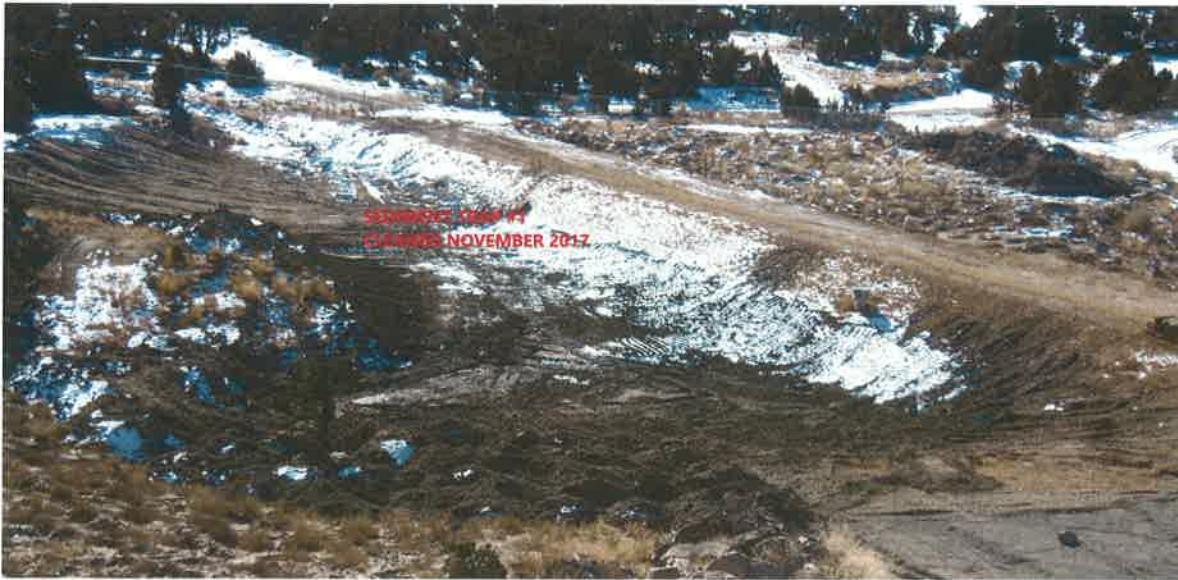
Sediment Trap #1, located immediately west of landfill – photo looking southerly January 12, 2018 Sediment was cleaned in June 2017 and again in November 2017
