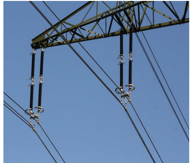
Fig. 22: I-Configuration Strain Insulators on Transmission Tower
