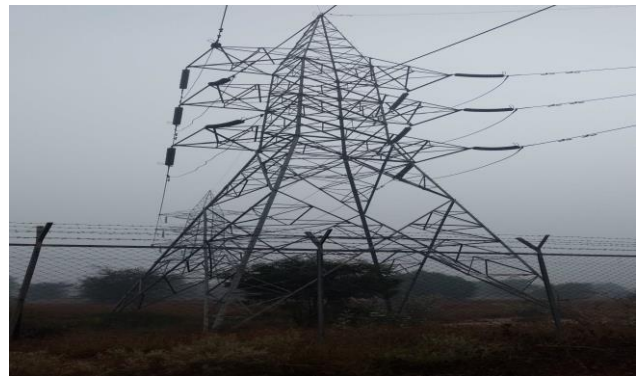
Fig. 13: Site of Broad Base Double Circuit at Nuiyanwali, Sirsa (Haryana)
