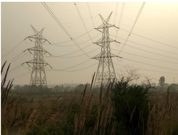
Fig. 6: Site of Broad Base Double Circuit (Multiple Conductor) at Sampla (Rohtak)
