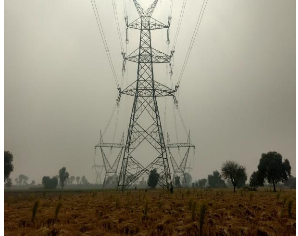
Fig. 7: Site of Broad Base Double Circuit (Three Phase) at Mayer (Hisar)
