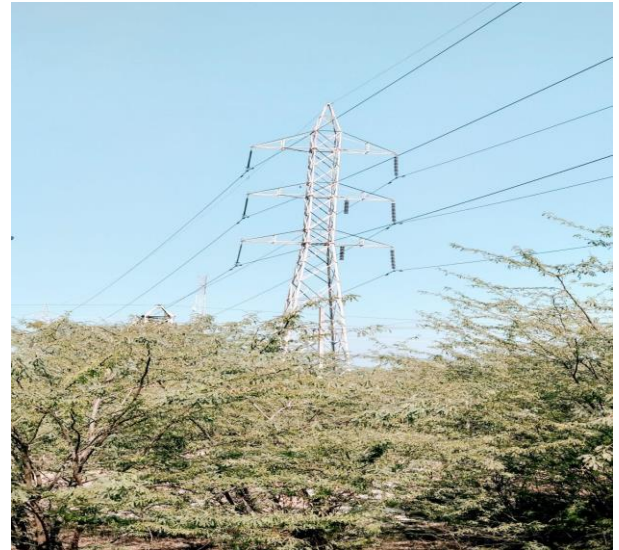
Fig. 4: Site of Single Circuit Broad Base Double Circuit at Dabwali (Haryana)
