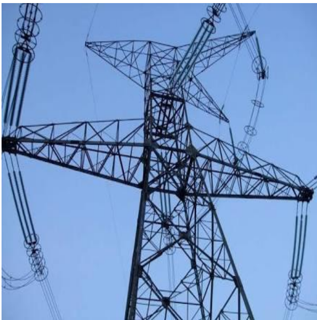
Fig. 19: Strain Insulator captured for Transmission Tower of 220kV
