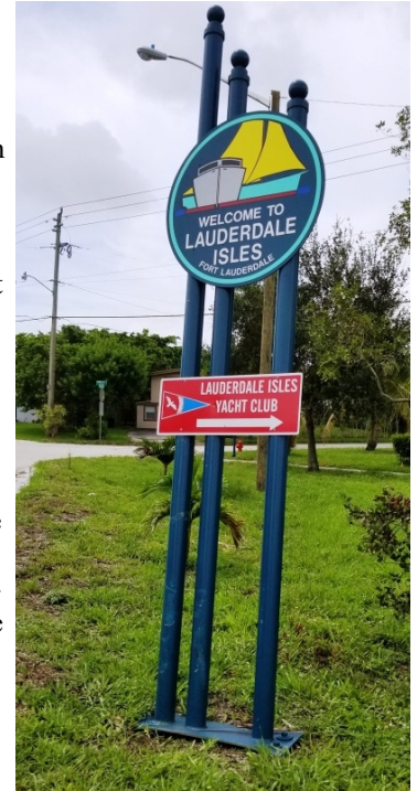
A bent metal base & cracked concrete footing by a hit & run on June 13.
