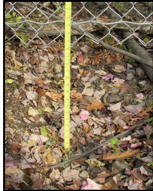
Large gap in perimeter fence at Boire Field
