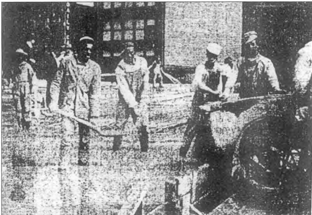
Figure 23: Wilkins building construction, African-American construction workers shovel concrete in pouring the second floor, view southeast
