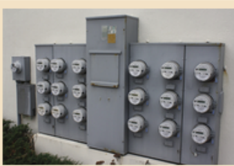
A bank of smart meters is pictured affixed to an Ocean City condominium building this week. Photo by Shawn Soper
