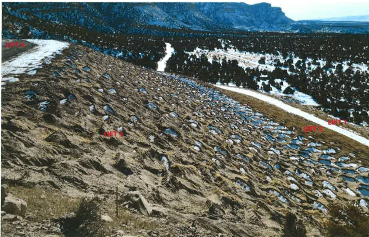
SCA#2 Ash Landfill – west face looking southerly Lift #1, #2 and #3 covered and seeded. Lift #4 in process
