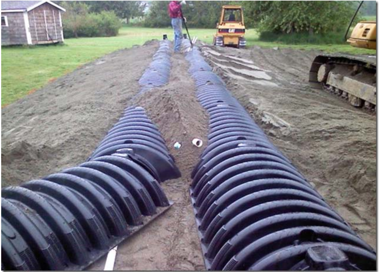
Installing CHAMBERS on the mound. Note the lateral piping under the chambers
