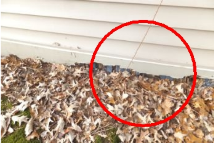
Rotting Siding on back of Storage Shed
