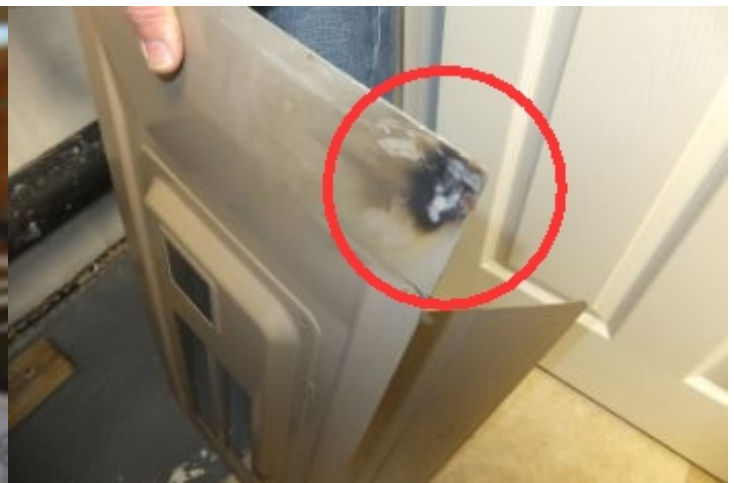
signs of arcing
