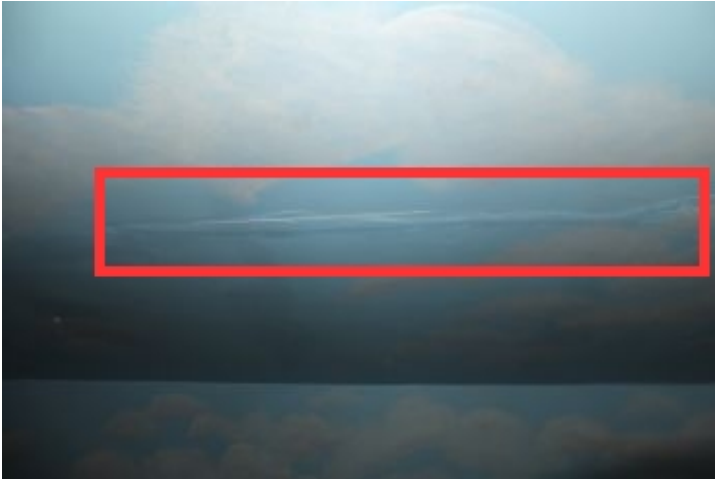
Bedroom 2 - repair needed on handyman work
