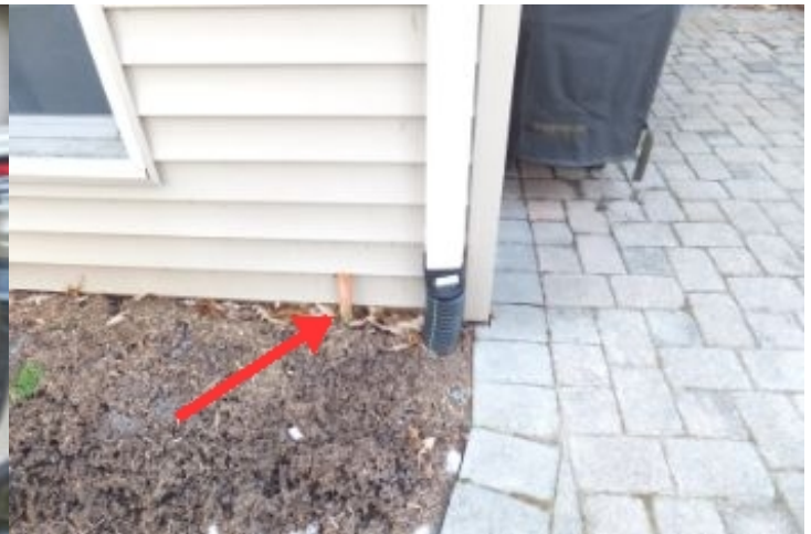
Evidence of treating for Termites
