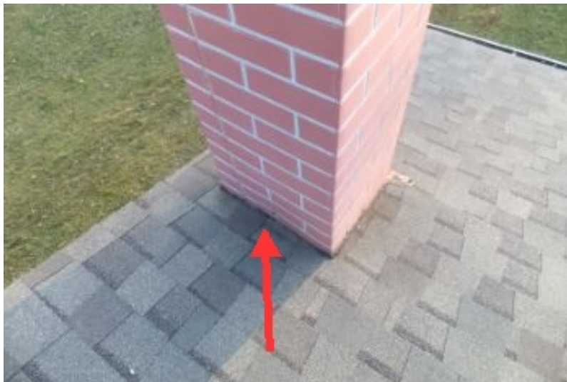
Missing backer flashing
