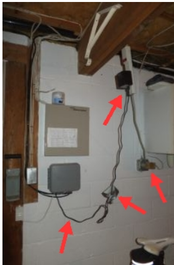
Sprinkler System plugged into plug strip
