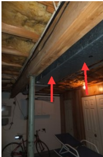
Supply Ducting not insulated
