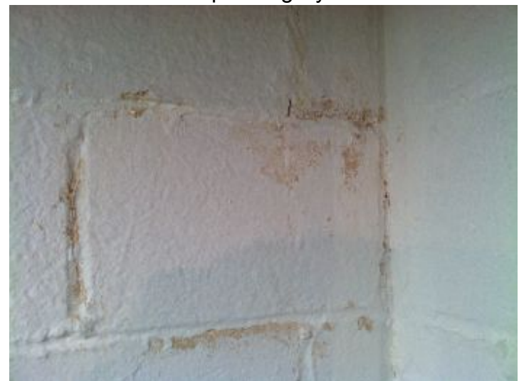
Water Stain on West Wall
