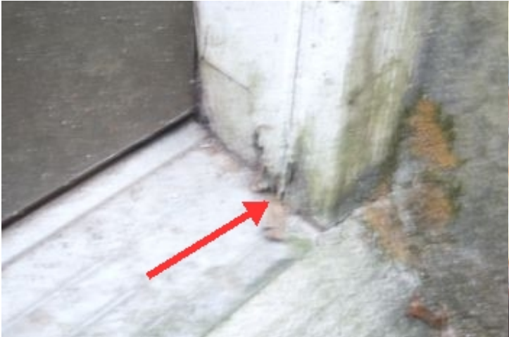
Door Moulding rotting
