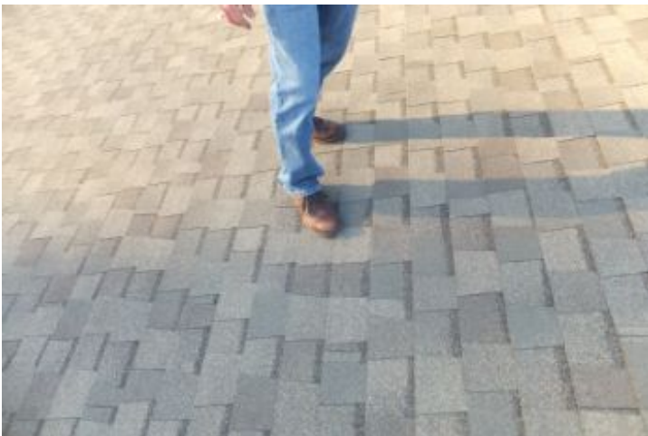
Soft Spot on Roof above foyer
