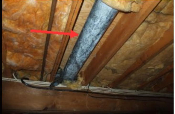
Supply Ducts not insulated
