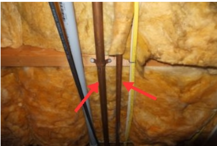
Water pipes too close together
