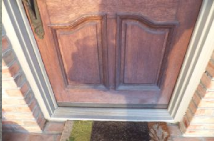
Front door is dry/peeling
