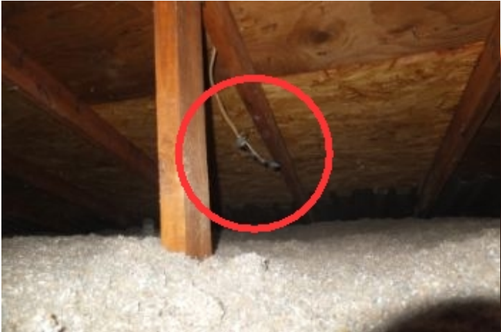
Open electrical conductor
