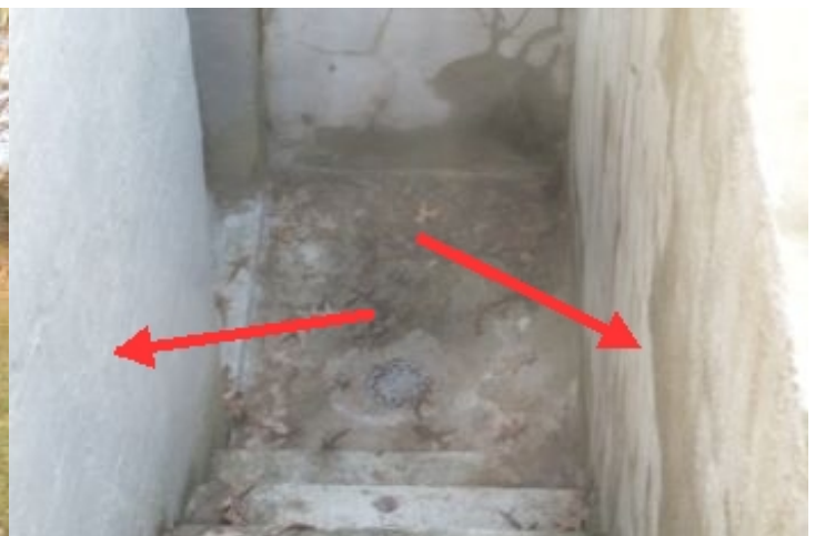
Basement Stair Well without railing
