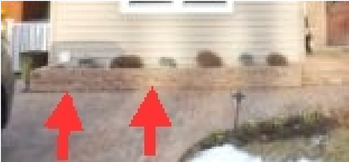
Flower Box without drainage could be directing water to basement wall
