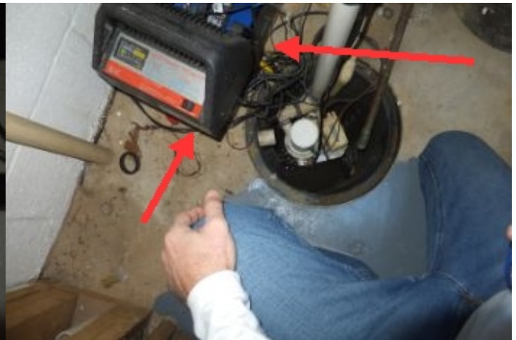
Sump Pump wiring with battery back-up should be off floor
