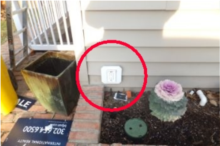
Cover Missing on GFI Receptacle
