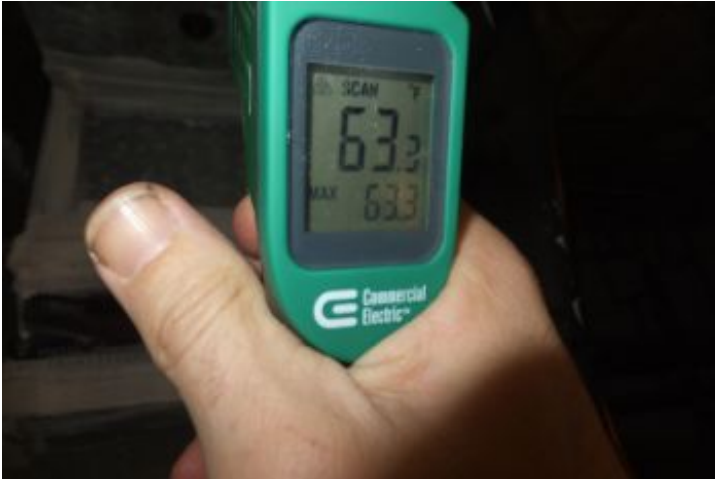
Supply Air Temp
