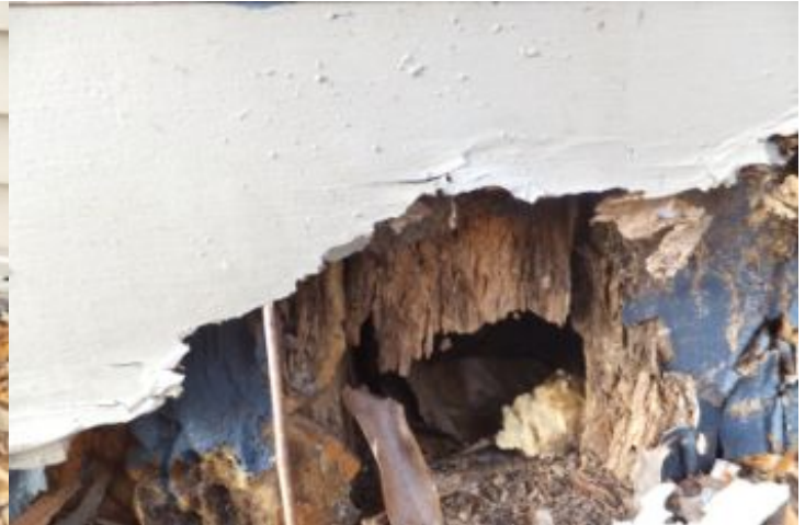
Rotting siding on back of Storage Shed
