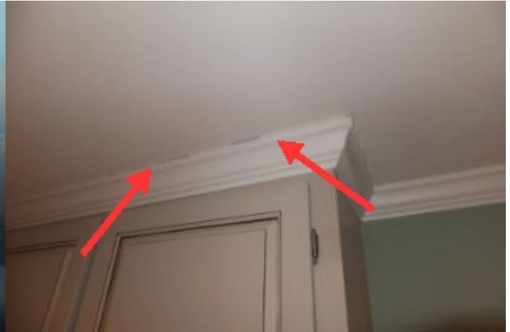
Some caulking needed in Kitchen
