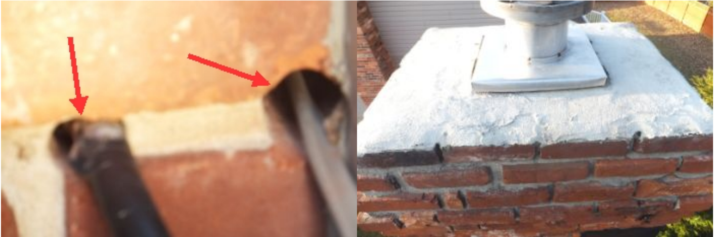
Gas line and electric cable not sealed
