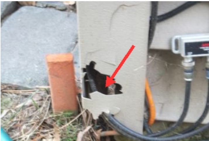
Cracked corner mold on siding
