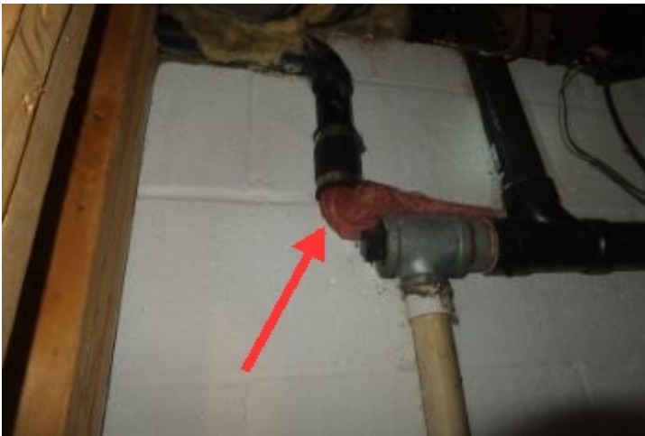
Sump Pump old drain pipe not capped
