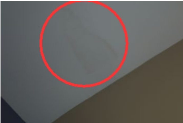
Water Stain on living room ceiling near fireplace
