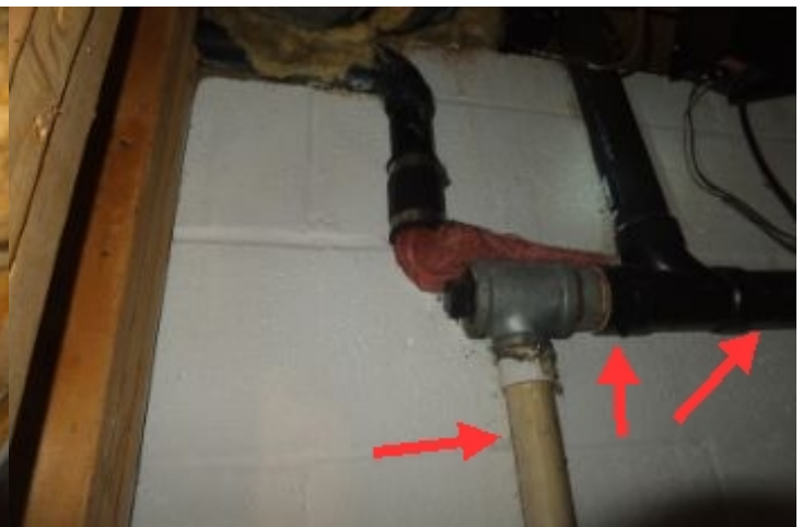
Drain to City Sewer
