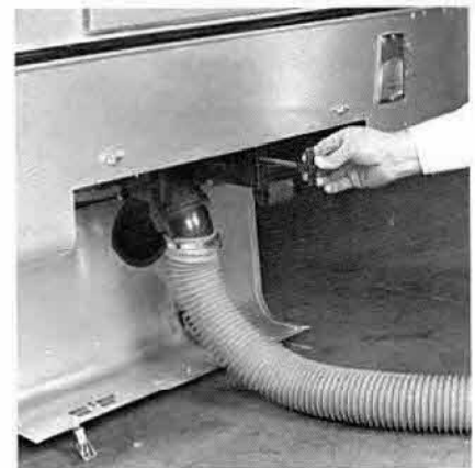
Waste Holding Tank Drain Valves
