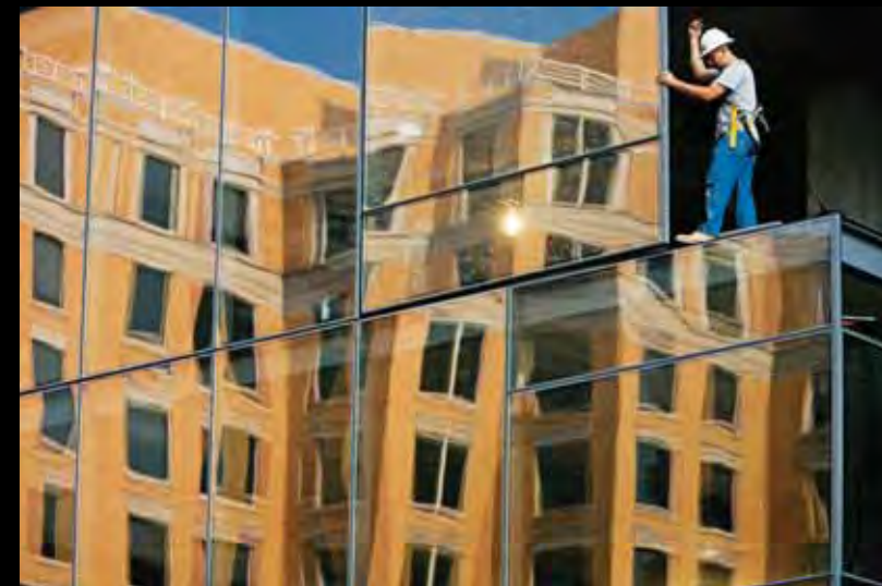
A worker in Washington, D.C., installs a triple-glazed window in a structure designed to meet strict "green building" standards. Advanced lighting, heating and cooling, and water systems, and a green roof contribute to a small carbon footprint, and can reduce energy costs by up to 75 percent. But many firms hesitate to invest in efficiency if up-front costs seem too high or payback times too long.
