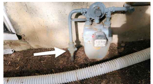
Gas shut off
