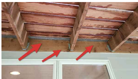
Missing lag screws
