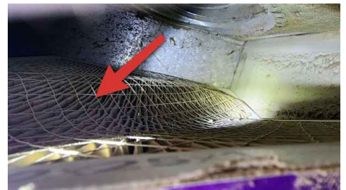
Replace dirty filter
