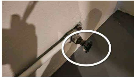
Basement shut off
