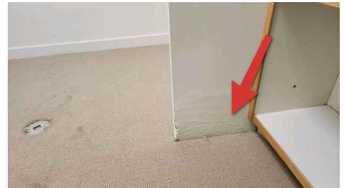
Old water damage
