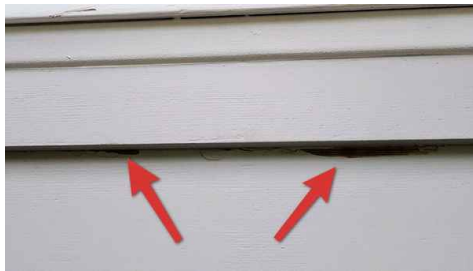
Peeling paint front of house
