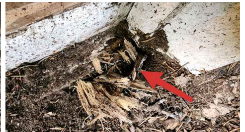
Rotted window trim
