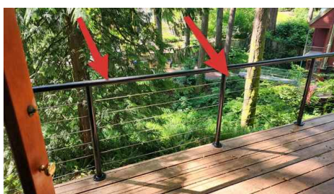
Balcony guardrail loose
