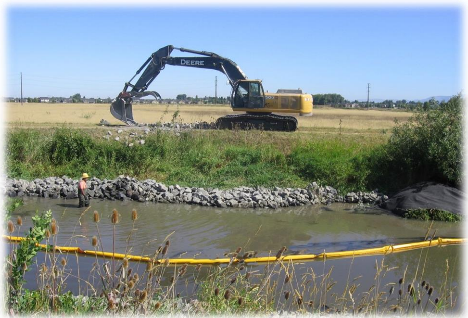
In areas where slumping or toe-cutting is problematic, such as the Amazon Creek Diversion Channel shown above, the City places rip-rap along the toe of the bank to limit further erosion. Bioengineering techniques, such as willow staking, are utilized where feasible to further stabilize the banks.
