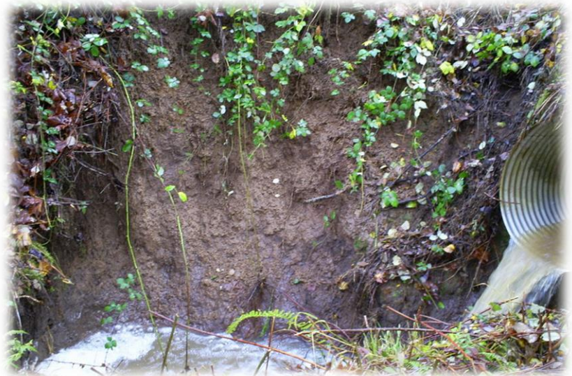
Incision along a headwater stream below an outfall
