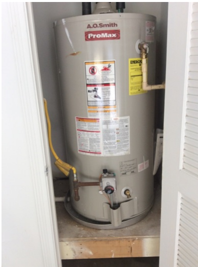
50 gallon, natural gas, in garage closet
