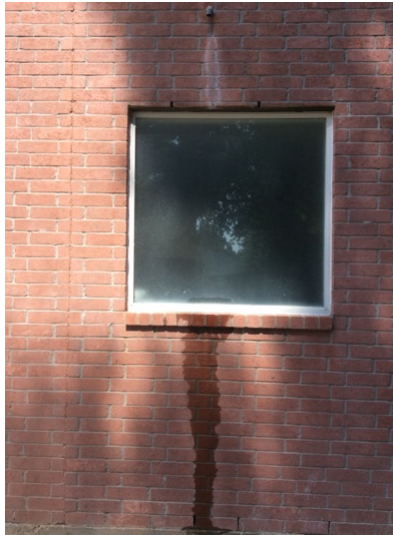
condensation draining from auxiliary pan drain
