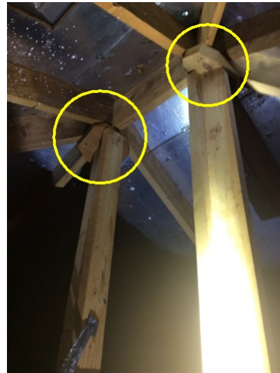
A framing shortfall uses these palm braces to make up for a mistake in the framing, an accepted industry practice
