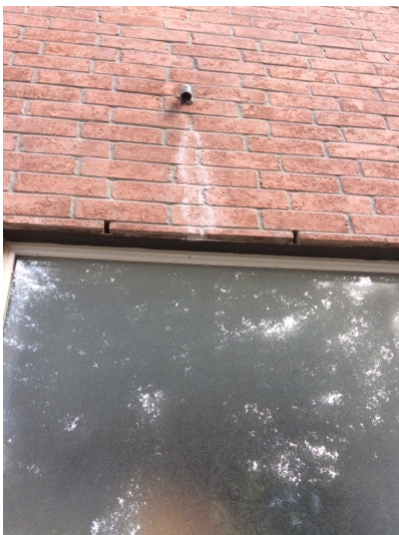
East Wall, driveway side, shows evidence of water drainage from AC secondary pan
