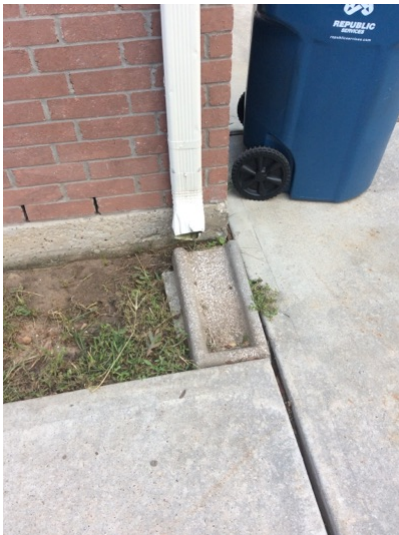
Throughout, drainage blocks all installed backwards
