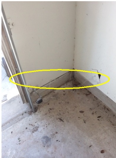
Sensor wiring requires repair
