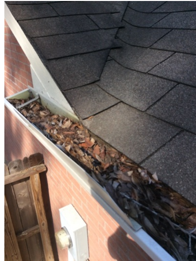
Gutters holding debris
