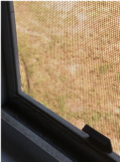
upstairs back bedroom screen requires repair
