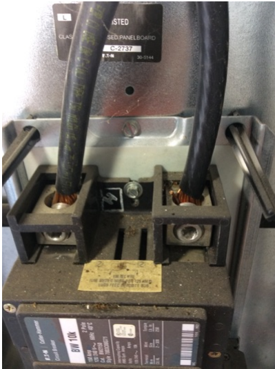
Service Conductors are Copper
