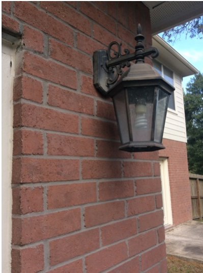
Porch light loose, requires tightening
