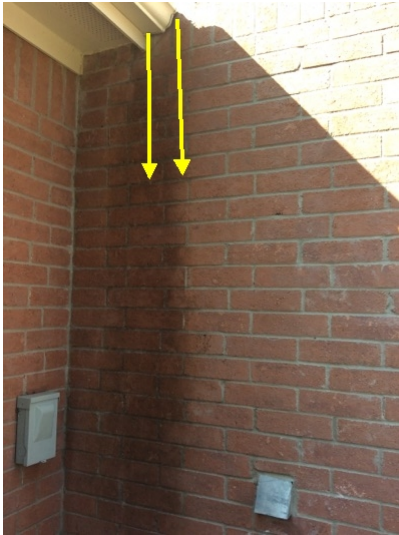
Gutter outside wall near fireplace drains water down onto bricks and AC slab, masonry moisture level very high
