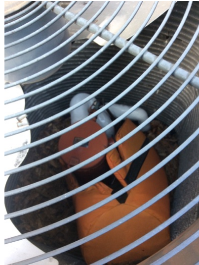
Frozen AC unit on inspection day
