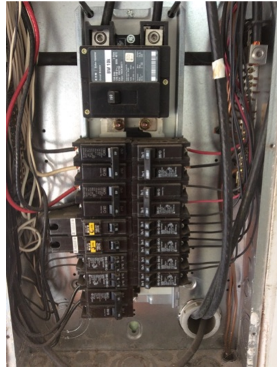
Cutler Hammer 150 Amp Copper service
