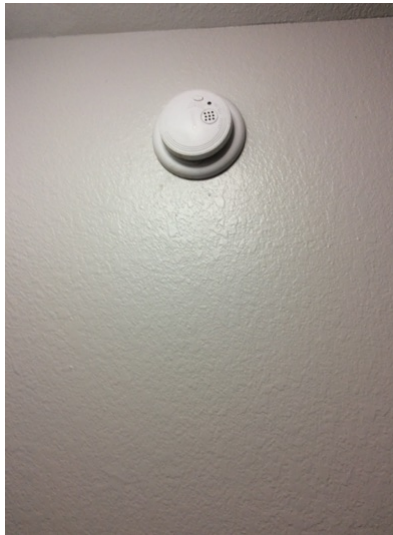
Two upstairs smoke alarms inadequate audible alarms, hallway and back bedroom
