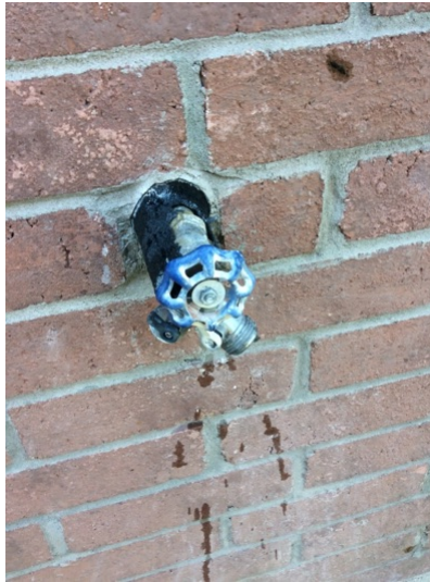
Throughout, outside hose bibs require new insulation covering
