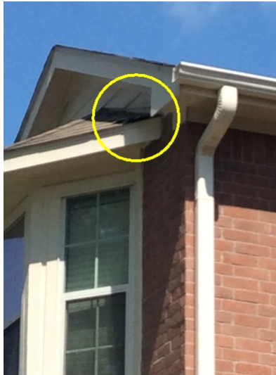
Front of home, roof requires repair to eliminate possible water intrusion
