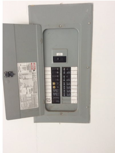
Cutler Hammer 150 Amp, in Garage
