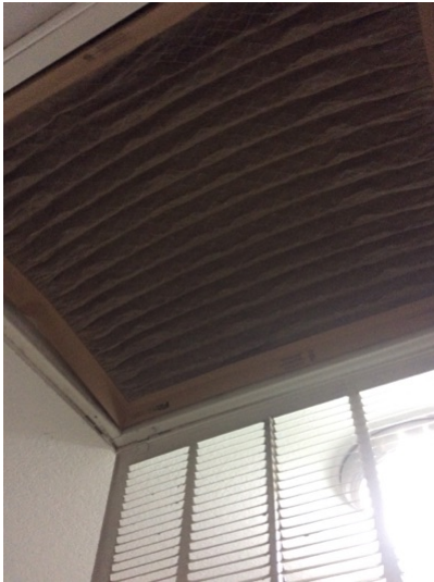
Hallway return air, requires replacement, sucking up into the duct air way
