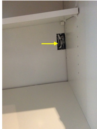
Open junction box inside kitchen cabinet, requires cover for safety
