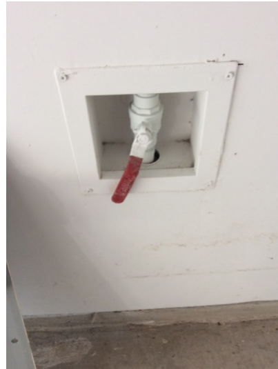
Main Water Cutoff Valve inside garage
