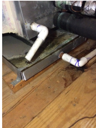
Condensate draining into auxiliary drain pan, requires maintenance
