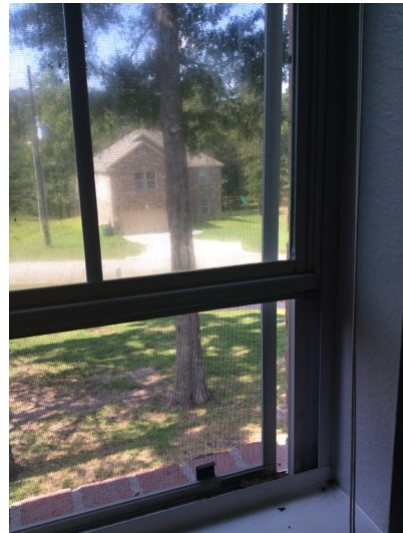
Stairway window screen fit not good
