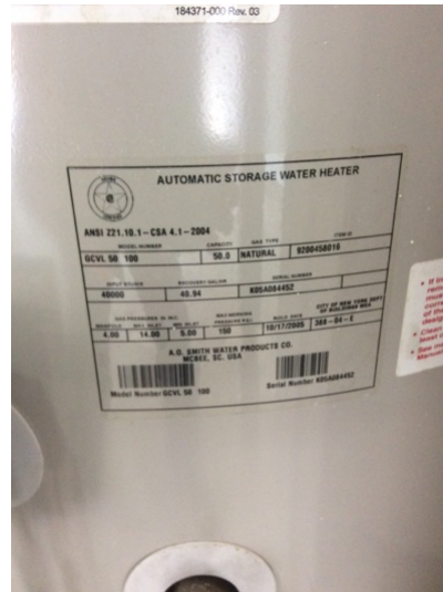
A.O. Smith Water Heater, natural gas
