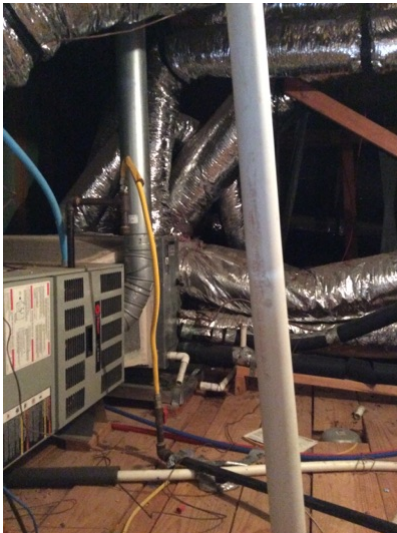
Ductwork in contact with one another causes condensation to occur
