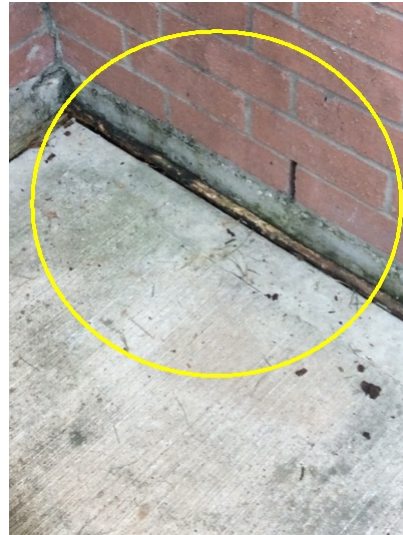
Wood decay from water above being spilled from gutter
