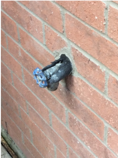
Outside Hose Bibs require new insulation covering
