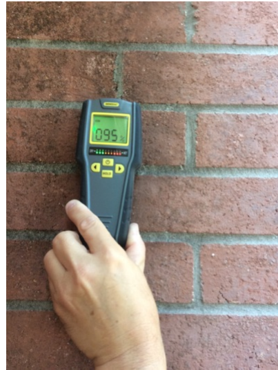
Gutter outside wall near fireplace drains water down onto bricks and AC slab, masonry moisture level very high
