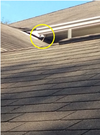
Upper gutter draining directly on to lower areas of the roof
