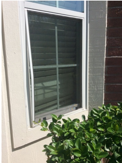
Downstairs screens damaged, require repair
