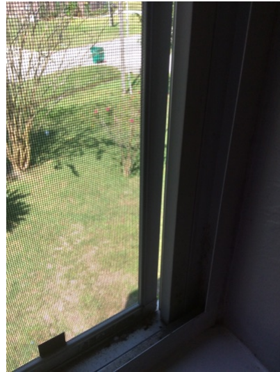
upstairs bedroom window screen requires repair
