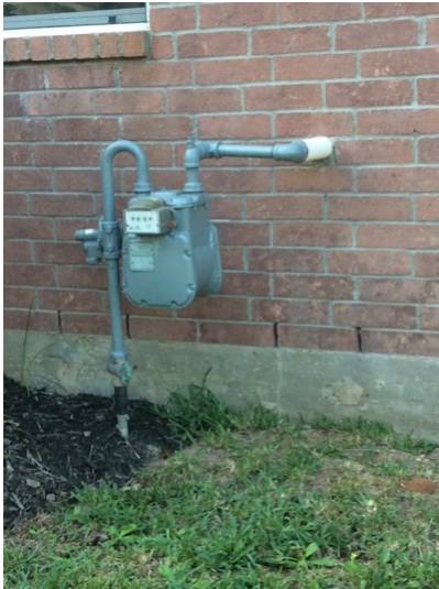
Gas Meter at North Side of Home
