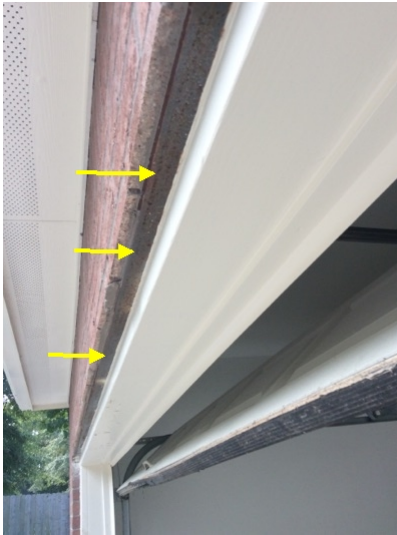
Lintels require annual maintenance, paint to avoid rust
