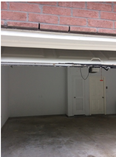
Garage Door Requiring Weatherstrip
