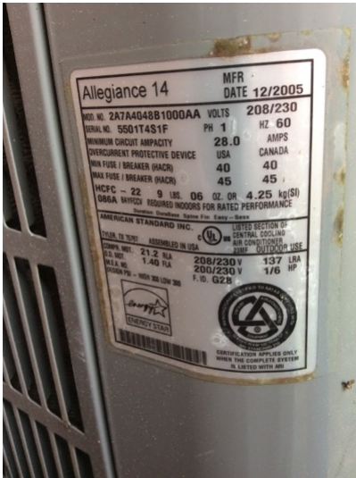
4 Ton, AC, Built December 2005
