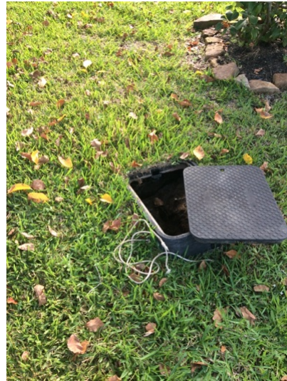
Water Meter South side of front yard
