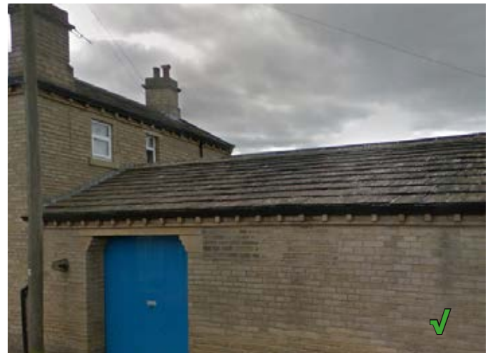
Single storey extension to building on Lee Green is subservient to the house and the detailing at the roof junction/eaves is good
